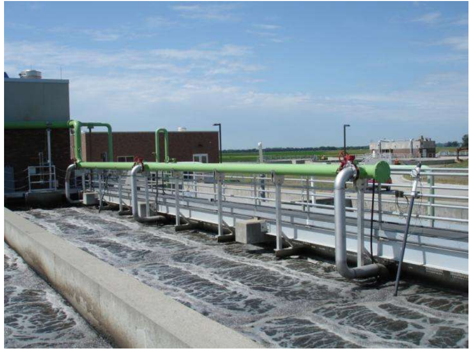
Photo illustrates west IFAS Basins in operation with Aeration Building and ABI Pump Station in background. Filtered effluent is pumped from the ABI Pump Station to the IFAS Basins and split evenly to all operating tanks. Photo shows green air header and individual 6-inch stainless steel drop pipes which feed air diffusers mounted beneath IFAS modules. Operators can monitor dissolved oxygen (DO) basin levels from upstream and downstream monitoring points in all four tanks and select desired DO probes for automatic blower control.
