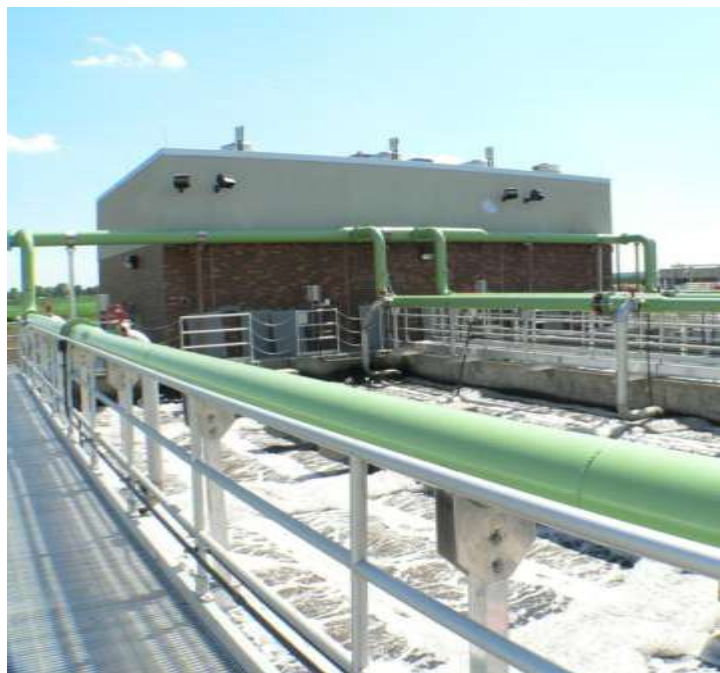
Photo illustrates the east IFAS Basins in operation looking south towards the Aeration Building. The green piping shows the 12-inch air piping header from the Blower Room and individual 10-inch branches to the IFAS basins. The new platforms are located to provide access to each basin and the associated air piping and control valves. The air piping was designed for easy access to air control valves and to accommodate expansion/contraction during varying operating conditions.
