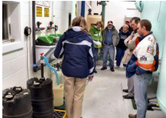
Laurie Twitchell, FOX Project Engineer, describes new chemical feed equipment to Mayor and Council Members
