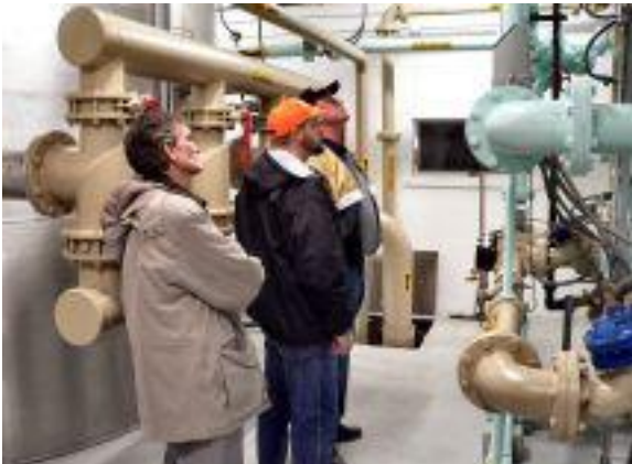
Council Members inspect automated softeners and new aluminum filtration unit.
