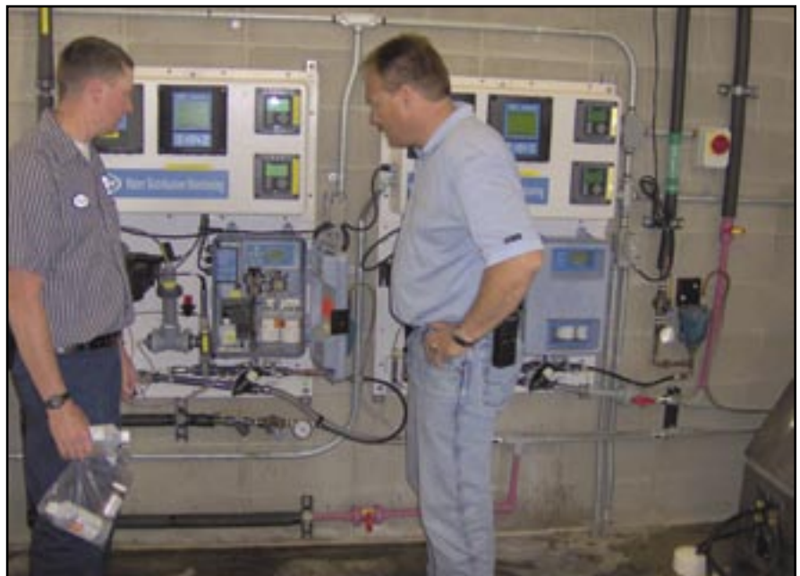
Wastewater Lab Manager Dennis Spilman (left) and Superintendent Kevin Moler inspect the Hach Water Distribution Monitoring Panels at the Clear Lake (Iowa) Sanitary District. Operators typically clean the sensors and check split samples against portable meters once a week.
